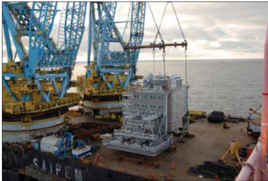
The Saipem 7000 crane barge lifted the new 455-tonne module onto the Snorre A platform (Fig. 1; photo from Statoil).
