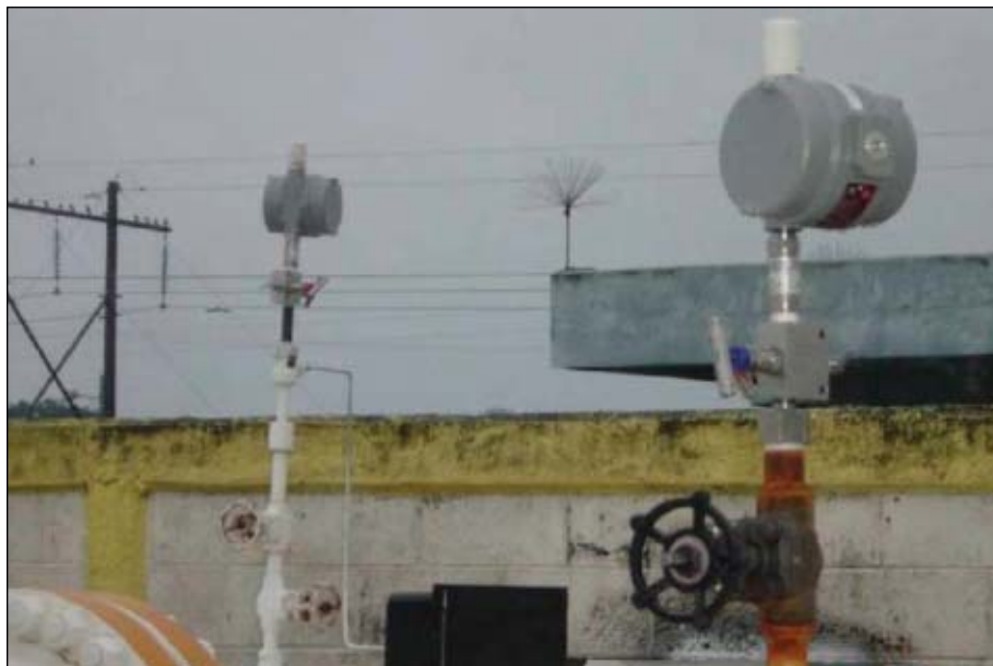
Wireless monitors such as these acquire operating measurements and convert these data into electrical signals suited for transmission over PGPB's existing communications network (Fig. 4).
